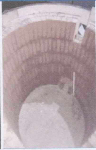
Cold Bricks Wall with HRTI 1200
