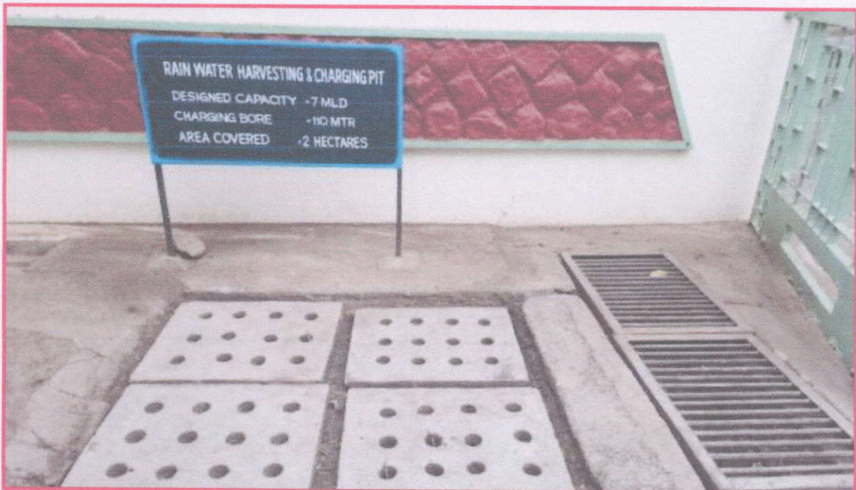
Sample Name Board in front a Rain Water Harvesting System
